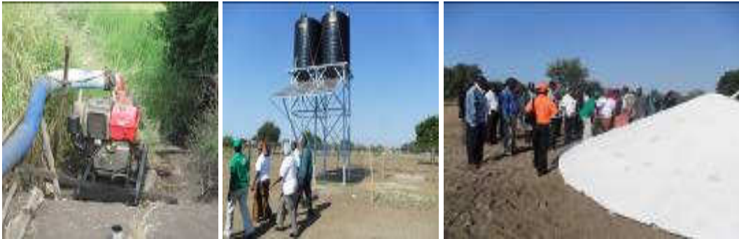
Picture 4: Water pump, Borehole systems with sun panels and water harvesting systems (April 2011 in – Nalazi, community, Guja district)
